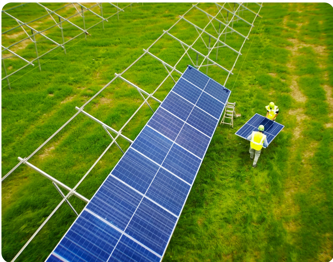
Plant installed at Finissaggio & Tintoria Ferraris S.p.A.
