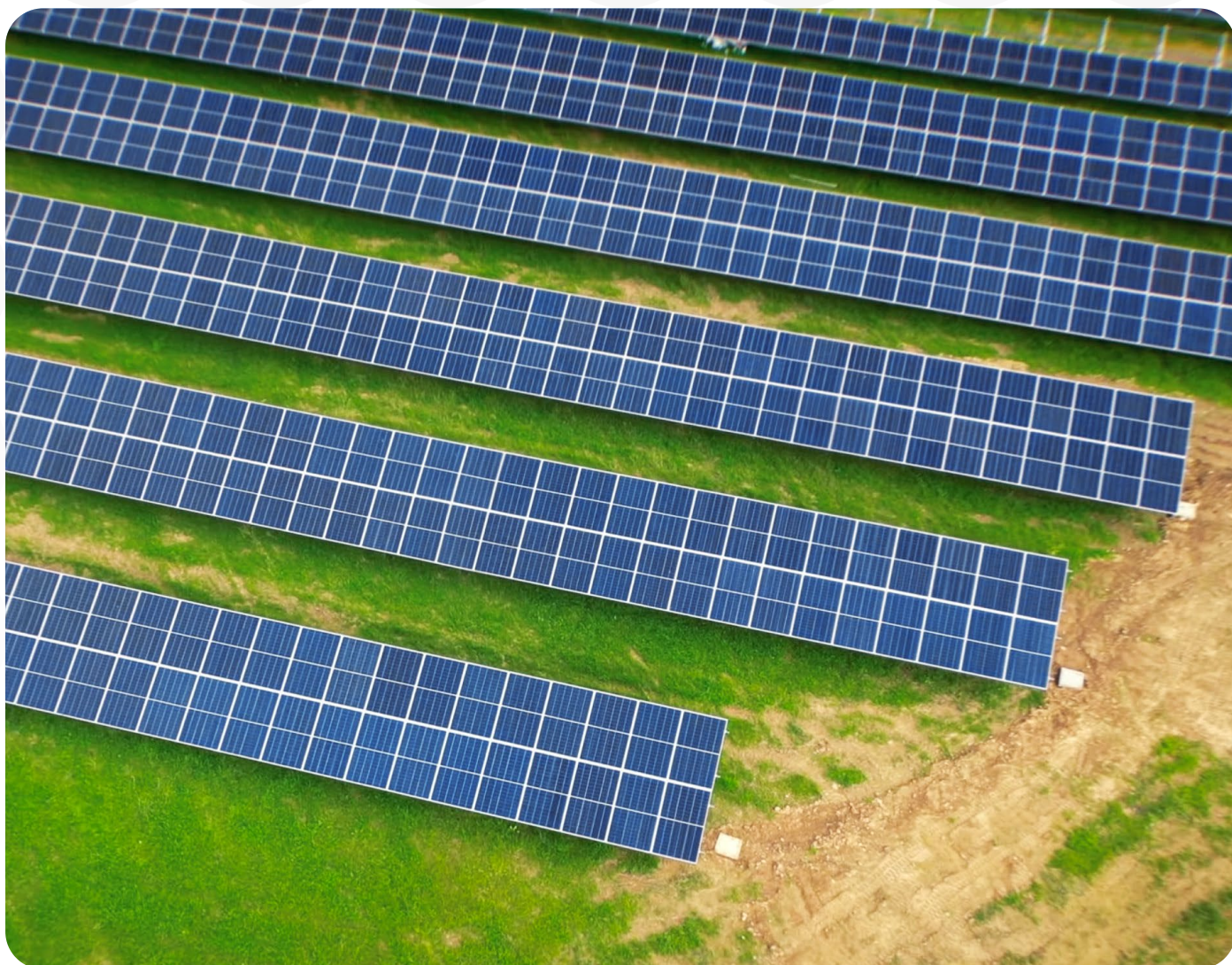
Plant installed at Finissaggio & Tintoria Ferraris S.p.A.
